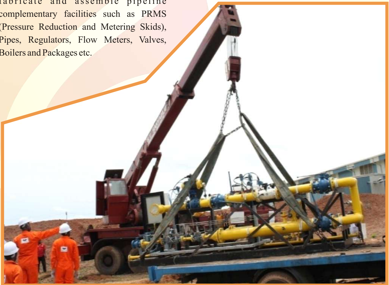
TOWER POWER 5MMSCFD PRMS
