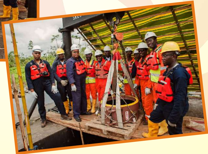
30" West Africa Gas Pipeline Leak Repair
